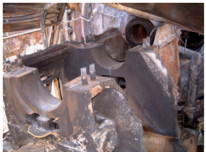
Figure 8: High Damage to surrounding equipment
