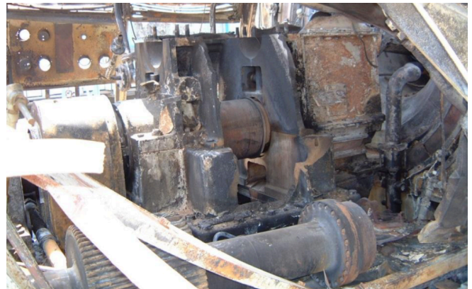
Figure 6: Gearbox explosion due to failure of bearing at load
